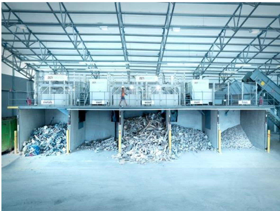
Figure 7: Overall photo of a ZRR
